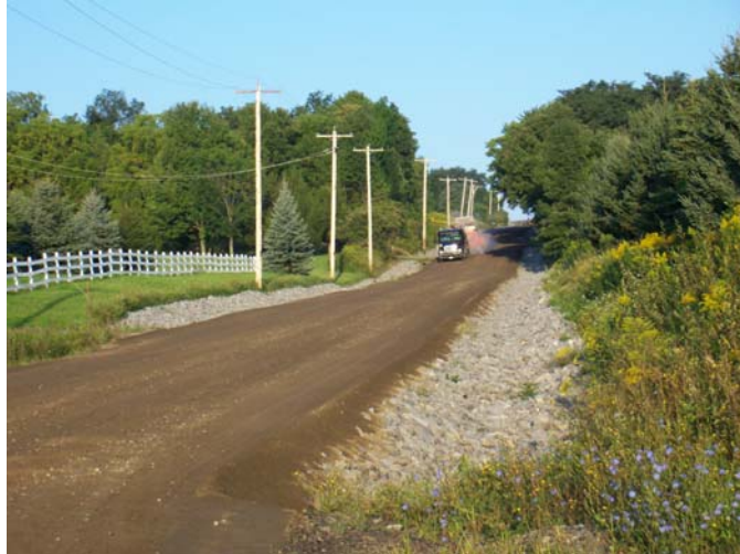
The ditches armored and new quality DOT approved Item 4 crushed gravel used as a base.
