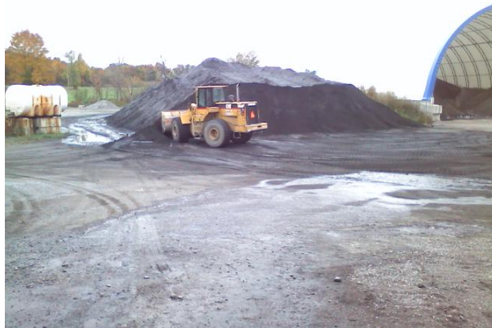
With the extremely rainy weather throughout August, our folks focused on hauling and stockpiling over 4,000 tons of cinders.
