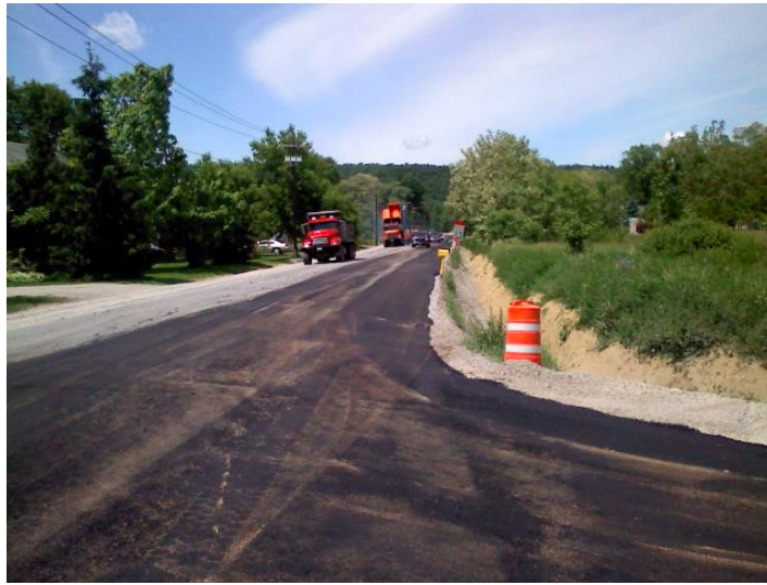
Conesus Highway working for the County Highway on Sliker Hill Road in July 2009
