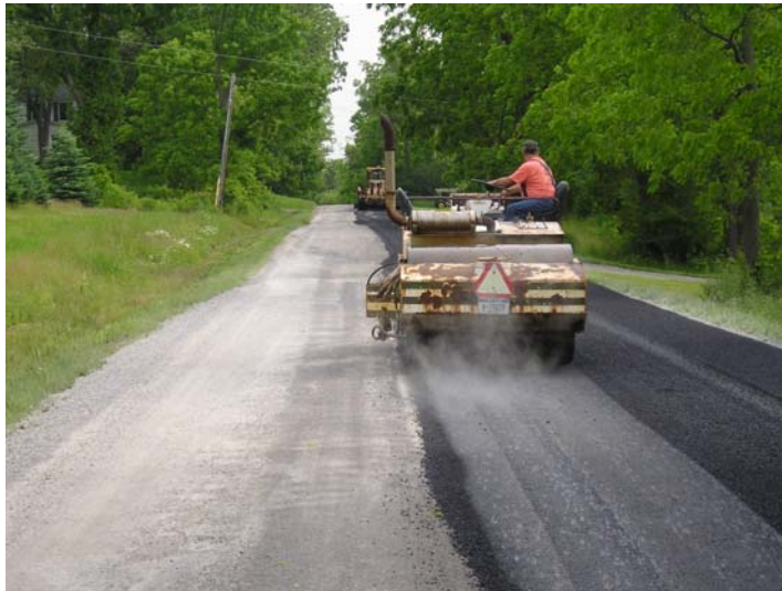
Repairing Clark Road with black top (wedging). John Clarke on the roller, July 2009
