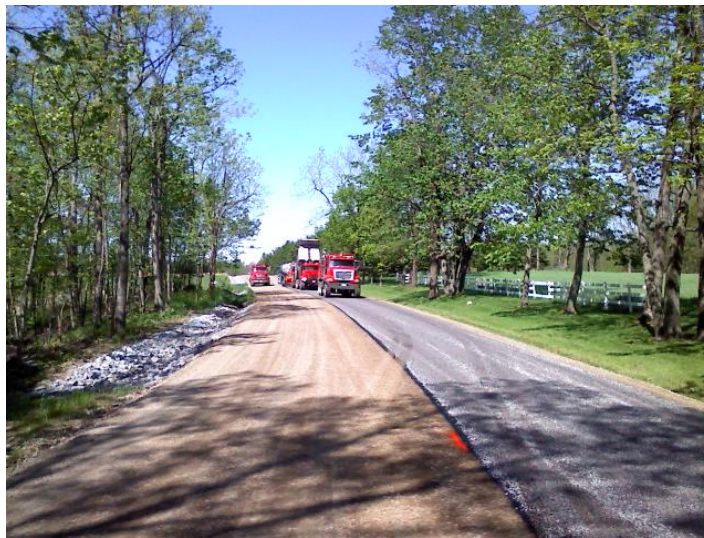
Oil and stone on Henderson Road in June 2009
