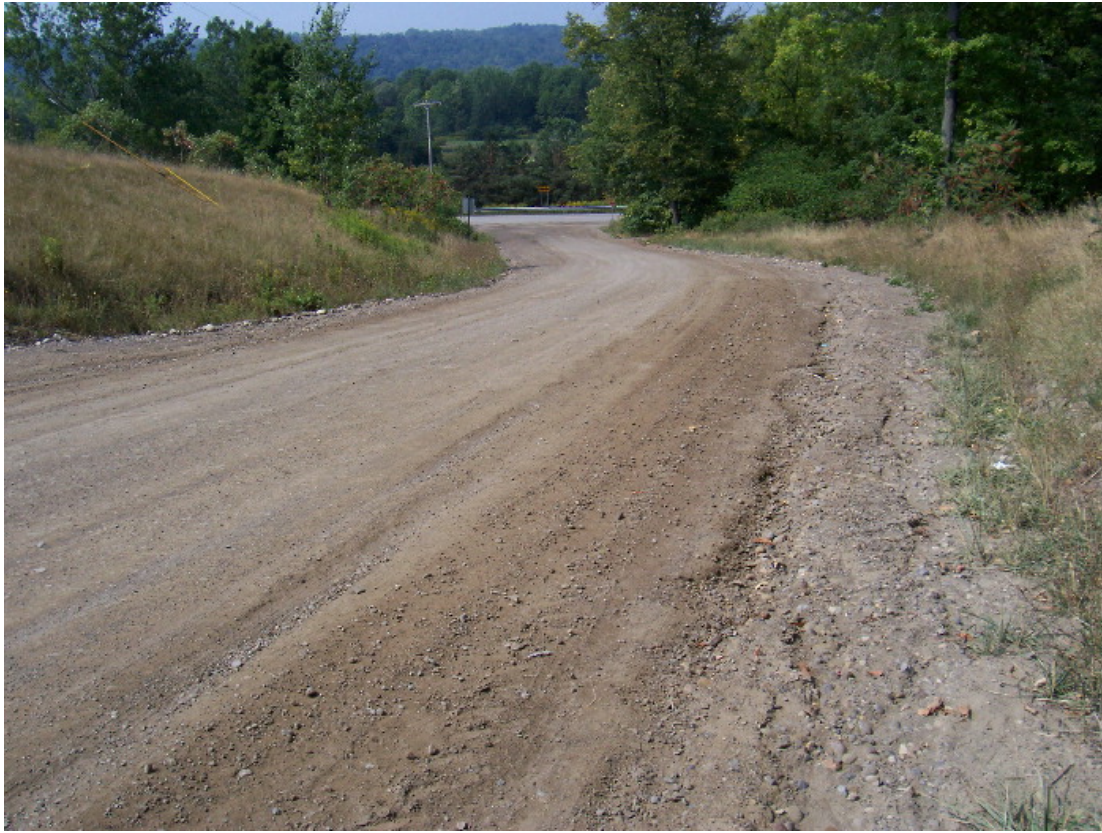
This photo shows the erosion problem (looking west). The East Lake Road is visible in the distance and Conesus Lake is just a few hundred feet further to the west.
