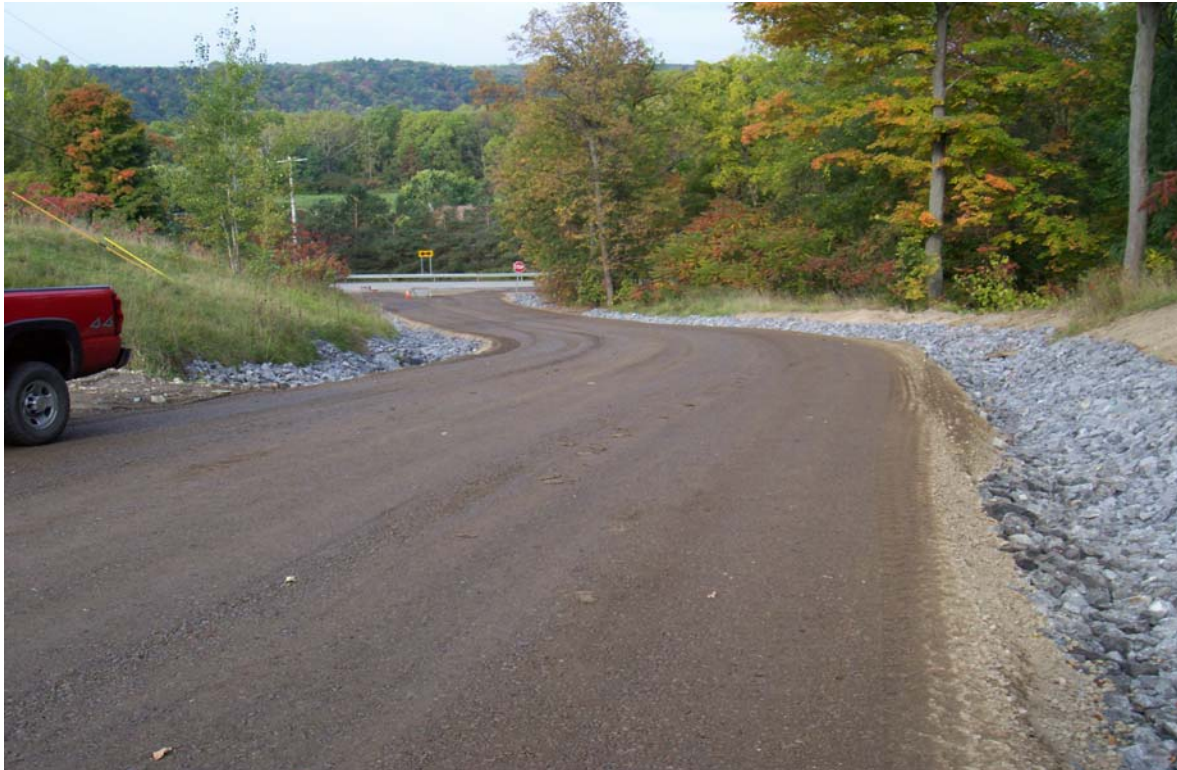
Taken September 2008, the roadbed finished and ready for oil and stone in 2009
