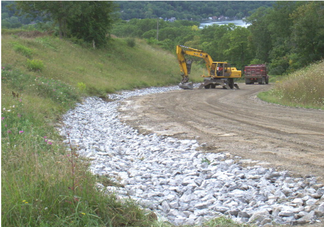
Although it appears that the new ditches are extremely shallow, the depth of the ditches includes over 3 feet of fill stone. Conesus Lake is visible in the distance.
